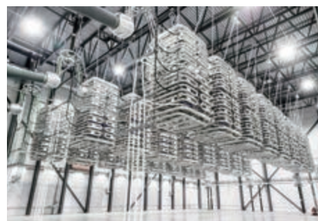
Ultra-high voltage gas insulated switching equipment
